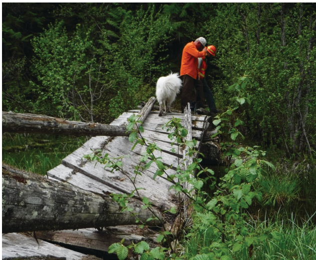
The North Fork Bridge Caused the Closure of the Red Bluff TR
