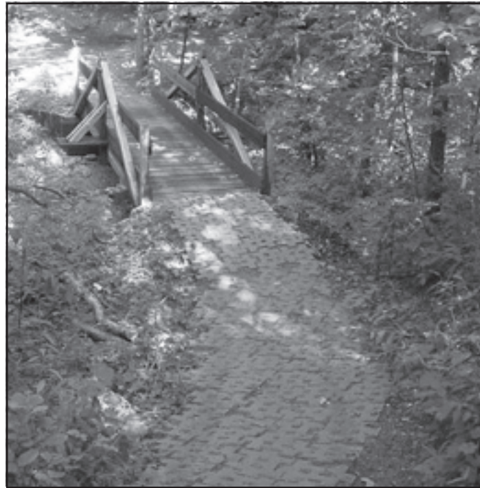
Figure 85—Pavers can be used to armor sections of trail for motorized traffic.
