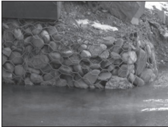
Figure 78—Wire baskets, often called gabions, are another retaining structure.
