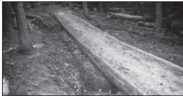
Figure 42—Turnpike maintenance includes recrowning the tread, cleaning out the ditches, and making sure the ditches are deep enough.
