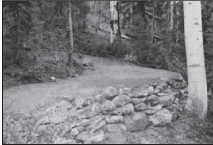
Figure 69—Part of the lower approach and the lower half of this switchback are constructed on fill.
