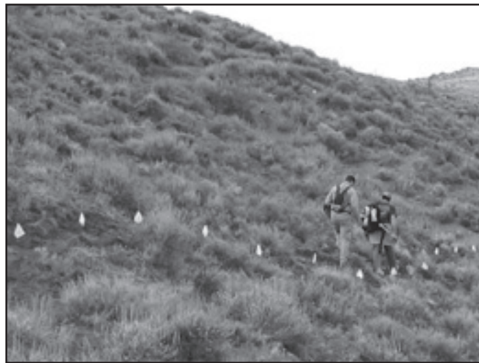
Figure 6—Pin flags mark the exact location of the trail tread and give you a good feel for the flow of the trail.
